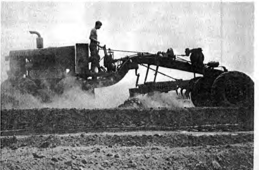
DRAGSTER -- Road graders were constantly employed by the 4th Engineers to tackle massive renovation projects.
